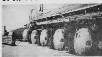
Making fresh water out of sea water is the continuous job of No. 2 Evaporator, above. Running constantly, it furnishes part of the water we drink. Over at the left of the picture is a tank built which has just been removed from one of the boilers. The whitish stuff is the lube-oil built up on the inside of the boiler which must be scraped off every day.
